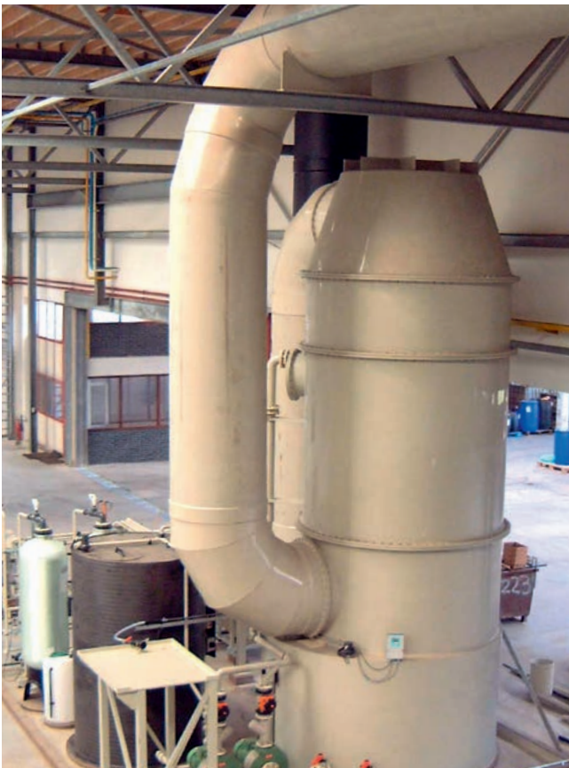
Exhaust air scrubber in PP
