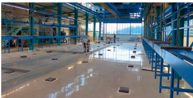
WHG coating of an impounding basin in a galvanizing facility
