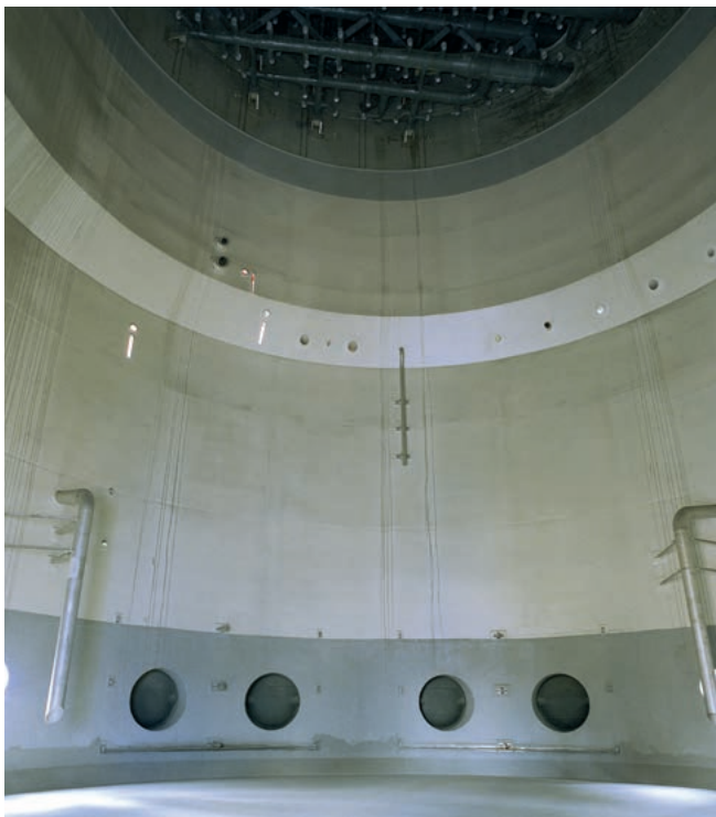
Lined flue gas scrubber
