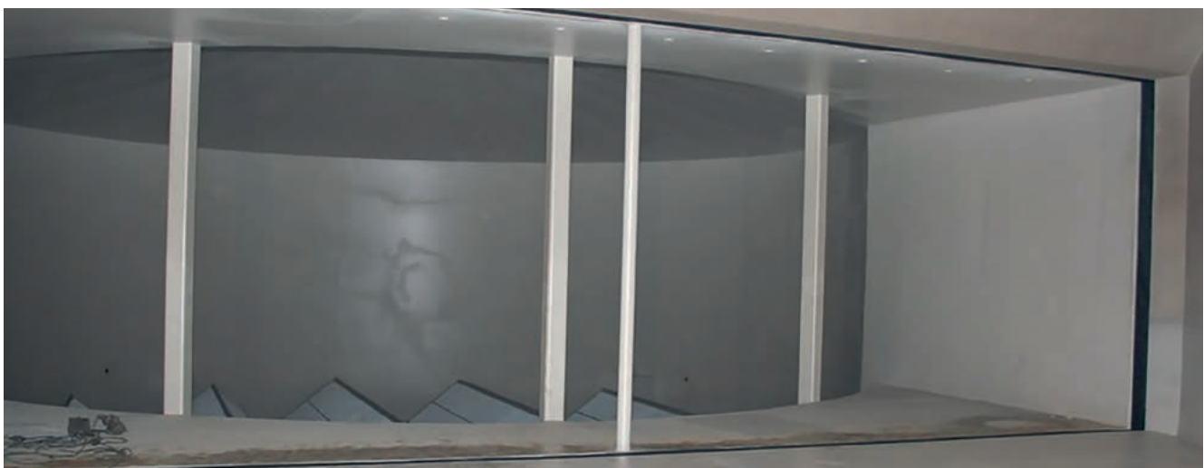
Coated clean gas duct
