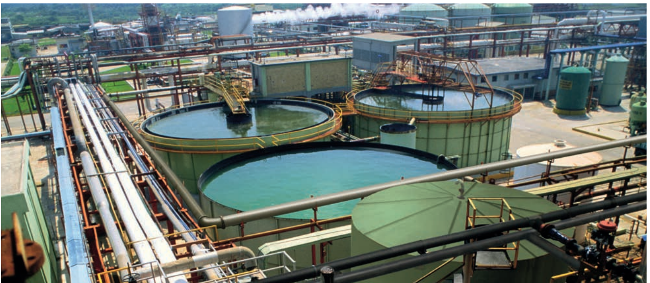
Rubber-lined sedimentation tank
