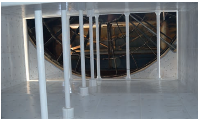
PFA lining in a raw gas duct
